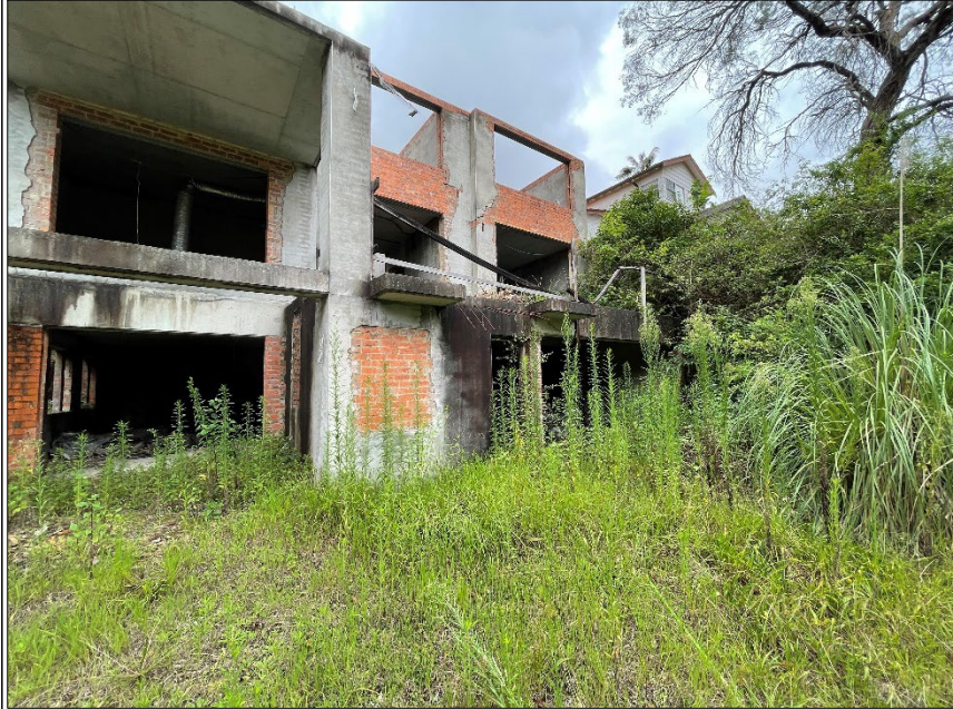
PHOTO 6: 17 HOLDSWORTH AVE, FACING NORTHWEST. CONSTRUCTION SITE APPEARS ABANDONED FOR A NUMBER OF YEARS.
